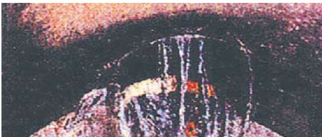
Water enters the manhole due to a pipe penetration.
