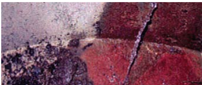
A crack at the base of a manhole allows water to infiltrate.
