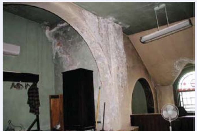
Fig 3: Distress in internal walls
