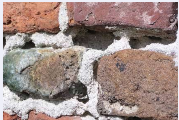
Fig: 3 Damage through salt Crystallization
