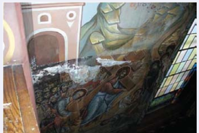
Fig 4: Damages in wall paintings
